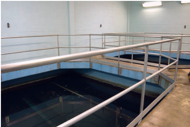
Water System Filtration Tank
